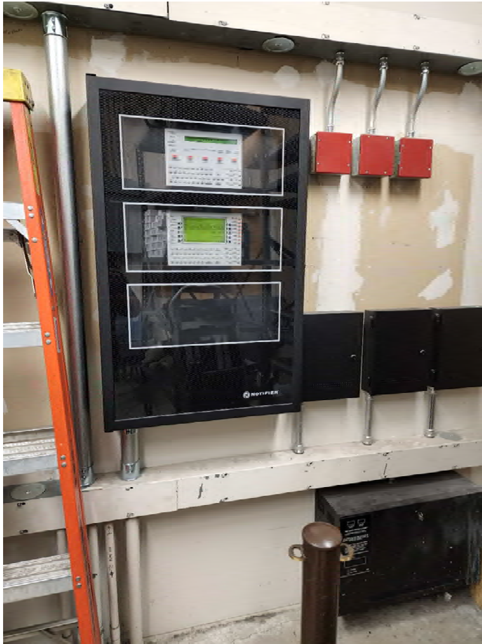
PHOTO FA1 FIRE ALARM CONTROL PANEL (FACP)
